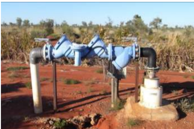
Figure 1 – RPZD Device, photo courtesy DEPWS
